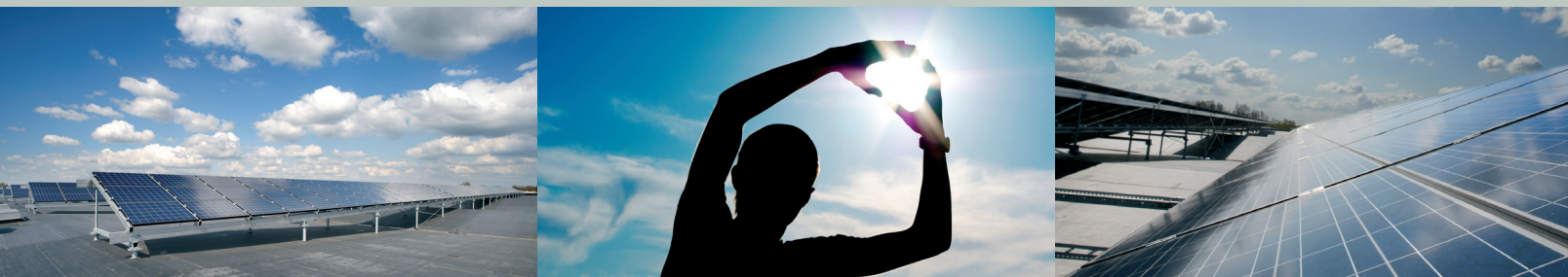
Reynaers - solar panels on roof of new distribution centre - Belgium
